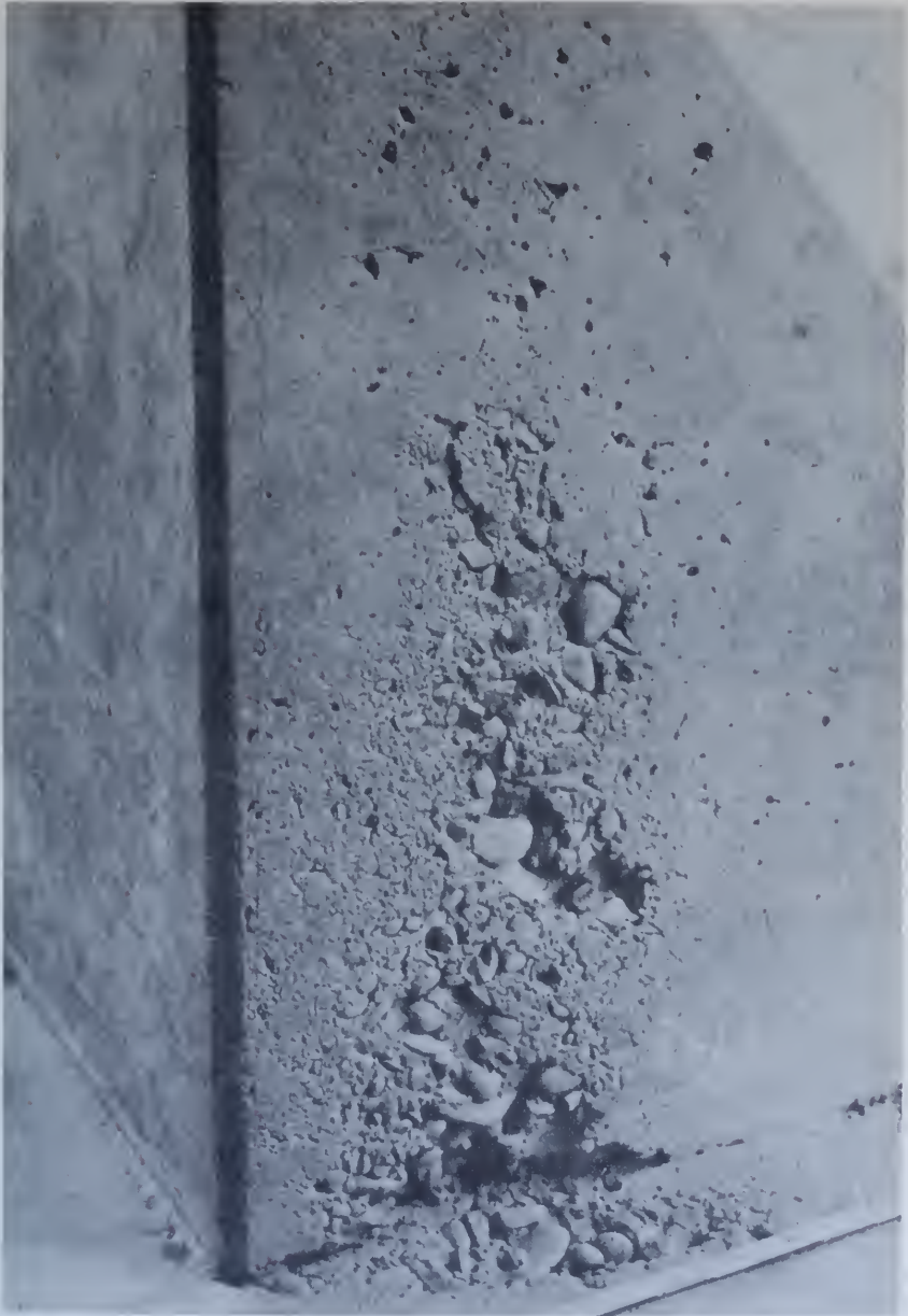
Figure 6.—Cavitation erosion of concrete on and adjacent to a dentate in the Yellowtail Afterbay Dam spillway stilling basin. Fast-moving water during a flood flow caused a pressure phenomenon at the concrete surface which triggered the cavitation damage shown here. P459-D-68902.
